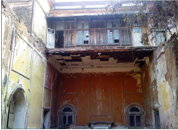
Figure 8. The Fallen Roof of Mubarak Manjil. (Source: Author)
