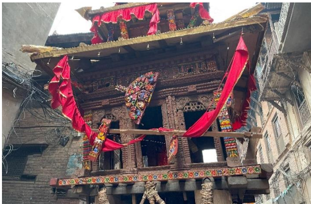
Figure 3. Dilapidated condition of the Bhailakha after the first day of the 2024 procession.
