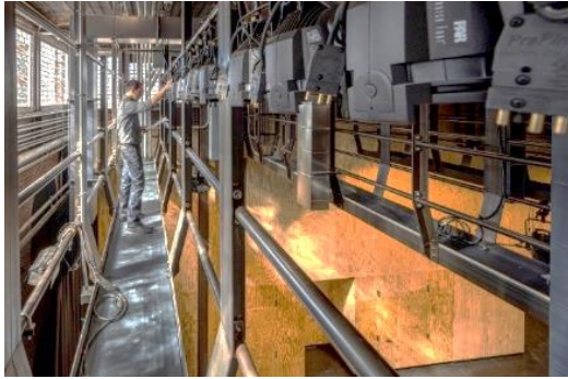
Figure 8. The overhead catwalk houses all technical elements and audio equipment, keeping the floor unobstructed and adaptable for a variety of functions.
