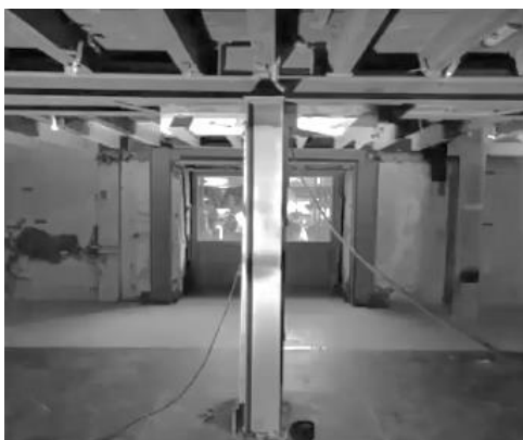
Figure 48. The condition of the ground floor when the building was acquired for transformation. Source: (n.d.). K Unwalla Architects.
