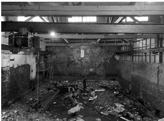
Figure 30. The dilapidated state of the ice factory post abandonment, with decaying walls and structural damage.
