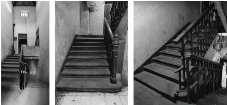
Figure 56. Photographs of the staircase before adaptive reuse – showing signs of sagging, vandalism, and neglect.
