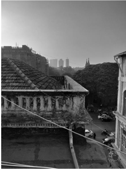
Figure 52. Dilapidated condition of the roof and Mangalore tiles prior to adaptive reuse. Source: (n.d.). K Unwalla Architects.
