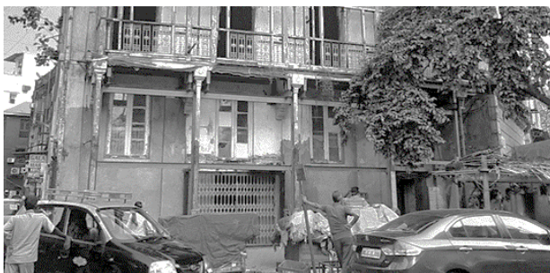
Figure 60. Damaged condition of the columns when the building was acquired.
