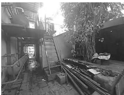
Figure 28. The courtyard before the adaptive reuse of the ice factory, cluttered with structures and debris that suffocated the banyan tree.
