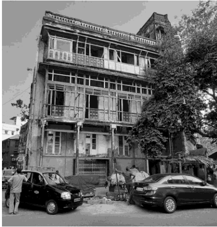
Figure 40. The condition of the Sassoon Building when acquired. Source: (n.d.). K Unwalla Architects.
