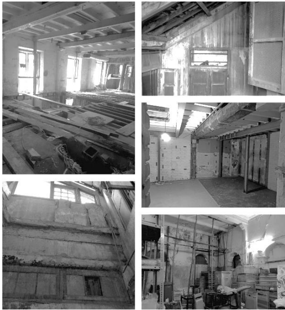
Figure 44. Images documenting the condition of the 165-year-old Sassoon Building at the initial stage of acquisition for adaptive reuse.
