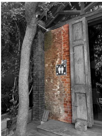
Figure 34. The wall facing the street reveals three distinct phases in the Ice Factory's timeline, each marked by variations in brick type and construction technique.
