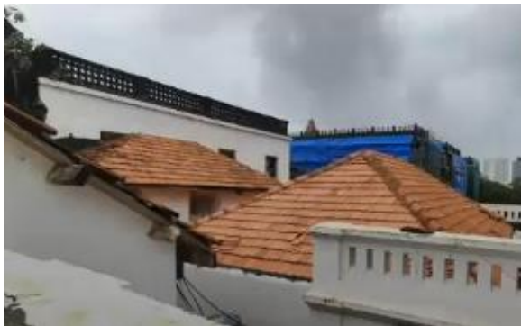
Figure 53. The roof post-adaptive reuse – restoration of Mangalore tiles and structural members revive the original architectural character.
