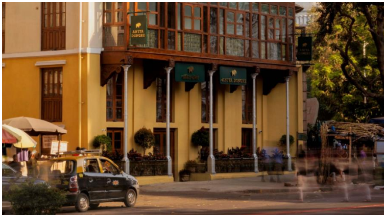
Figure 61. The structural columns supporting the balcony were salvaged, restored and enhanced by painting.
